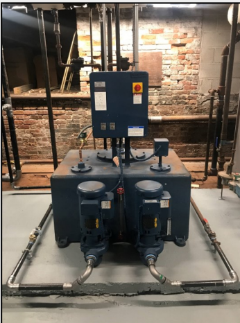
A new condensate and feed water tank was installed, serving both the Church & Cranmer boilers.
