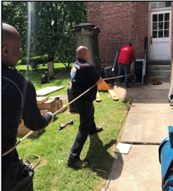
With strong backs and lots of muscle, 8000lbs of boiler are lowered into the basement
