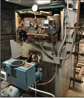
The old boiler was crumbling, leaking and at the end of its life.
